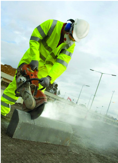
RCS exposure without dust suppression can be massive
